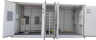
1075KW HH ESS
