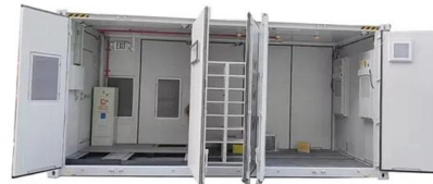
1075KW HH ESS
