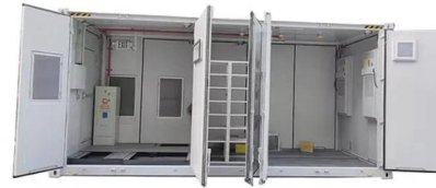
1075KW HH ESS
