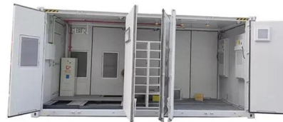
1075KW HH ESS
