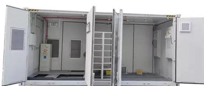
1075KW HH ESS
