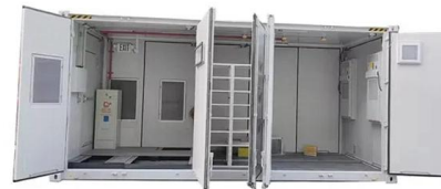
1075KW HH ESS
