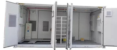
1075KW HH ESS
