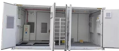
1075KW HH ESS
